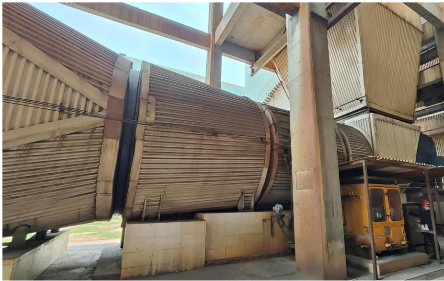
Figure 1 Physical induced draft fan monitored by the project
