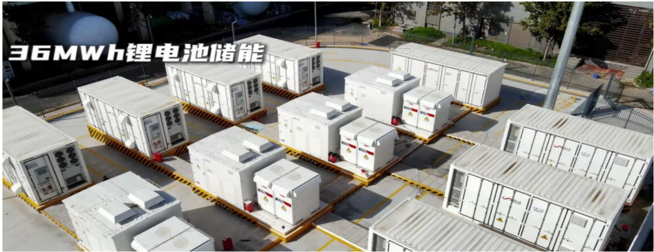
Figure 2 36MWh Lithium Battery Energy Storage System of Lingang AIDC
